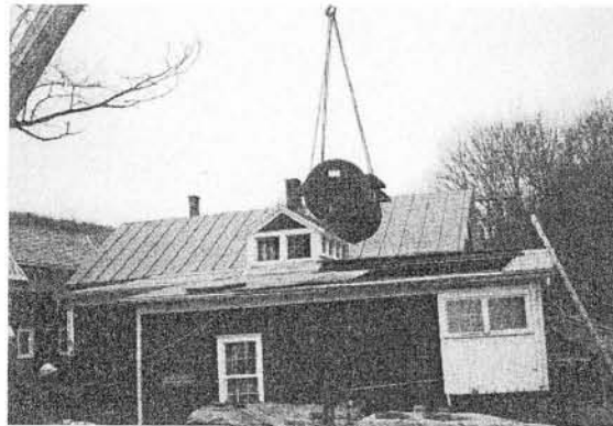
← 1. They have rigged the boiler to the crane and we're ready to lift!
